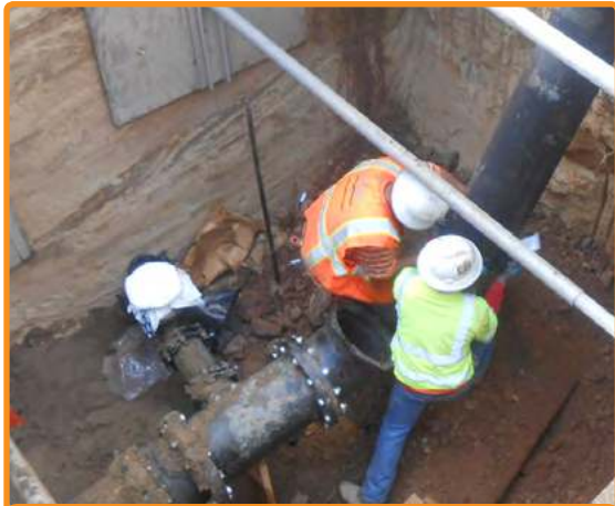
Construction crews work to replace a CHWD water main. These replacements are necessary to keep the system up to date and reliable.
