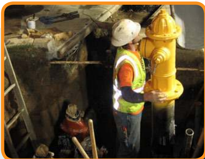
A crew member works in a trench to replace a CHWD fire hydrant. CHWD’s 271 miles of underground pipes not only provide water to homes and businesses, but also serve municipal needs such as fire hydrants.
