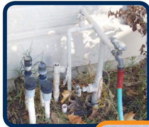
An uninsulated pipe is at risk of freezing and bursting during winter weather. It's also wise to unhook your hose during freezing weather.
