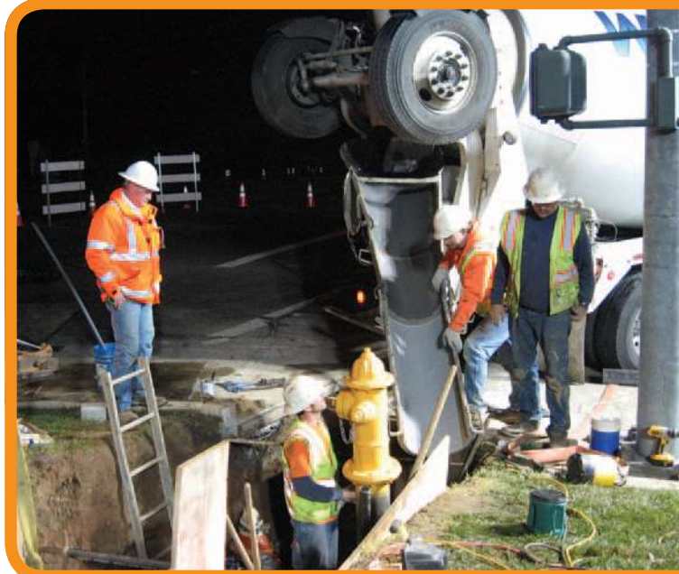
Construction crew pouring concrete as work on the water main replacement wraps up.
