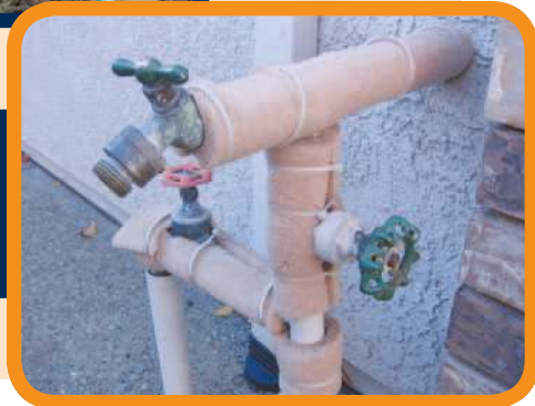
Insulating your pipes helps protect them from freezing weather conditions.
